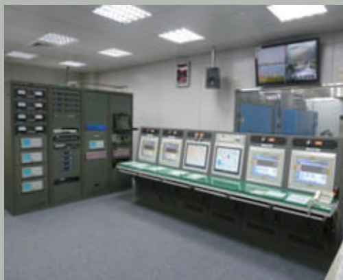
■ 控制室內部監控系統及成音設備 Monitoring and sound equipment in the control room
